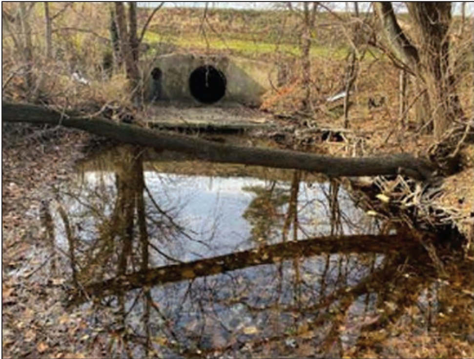
Photo 2: View of the Area of Concern (Phase 1), Abraham Faw Run Outfall and Existing Headwall Plunge Pool, facing southwest
