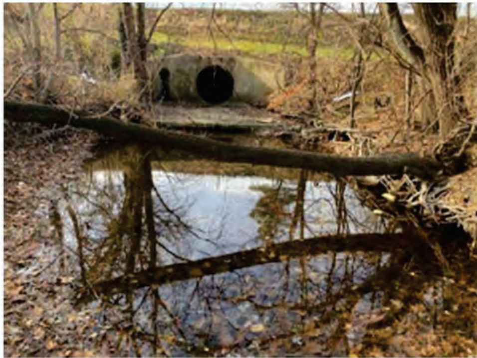
Figure 3. Photos of Abraham Faw Run Outfall and Existing Headwall Plunge Pool
