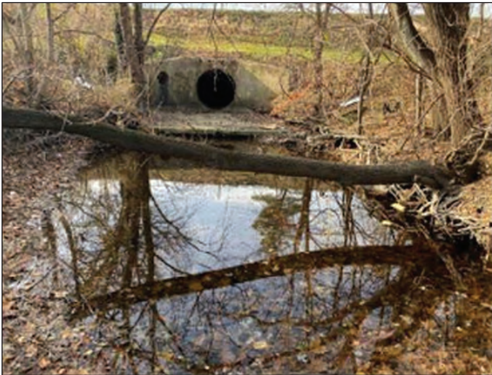
Photo 2: View of the Area of Concern (Phase 1), Abraham Faw Run Outfall and Existing Headwall Plunge Pool, facing southwest
