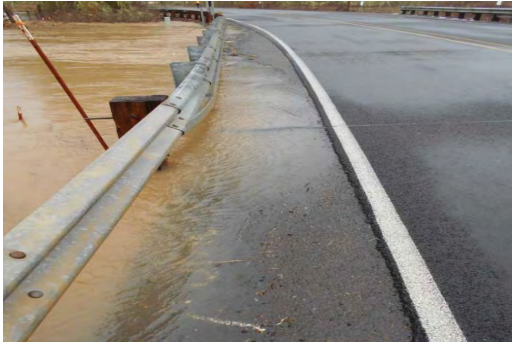
Figure 7: Flooding along the western roadway shoulder at north bridge (04057A) resulting in the erosion of the roadway shoulder
