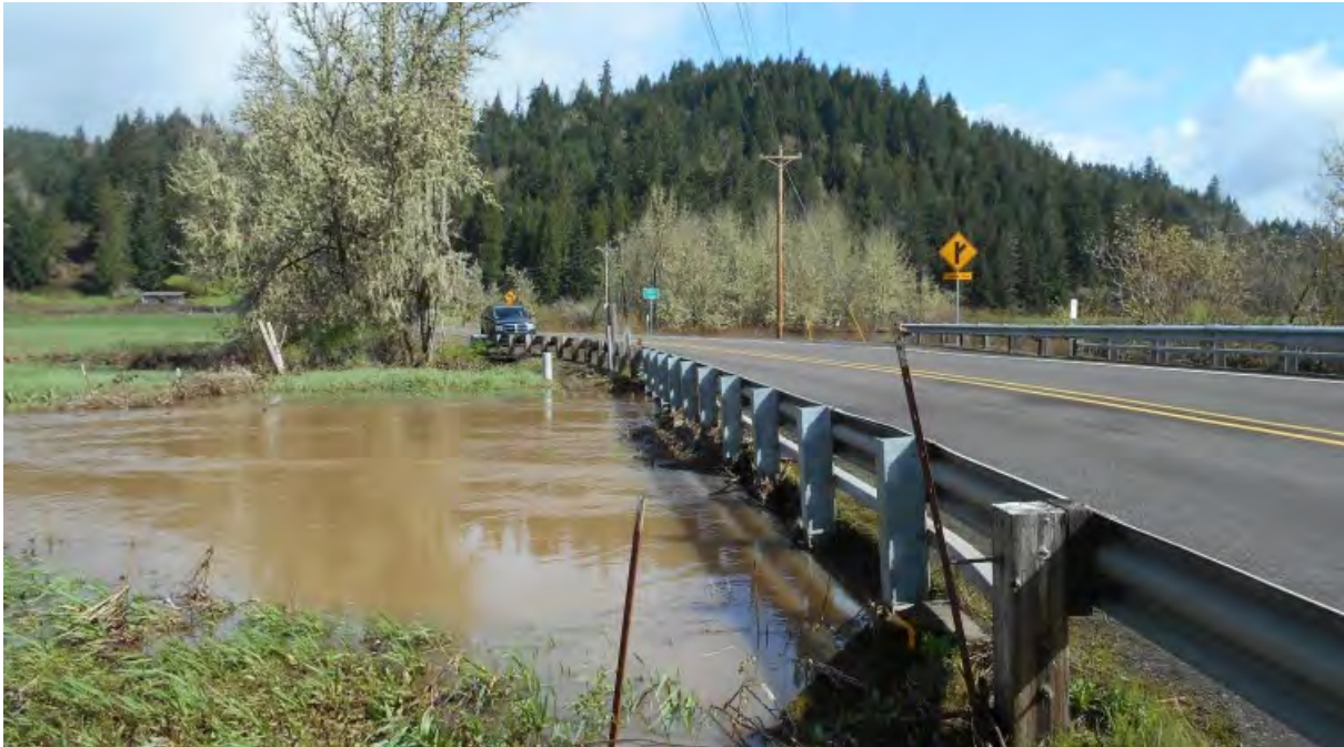
Figure 5: View of the existing north bridge (04057A) that traverses Coyote Creek during a flood event in April 2019
