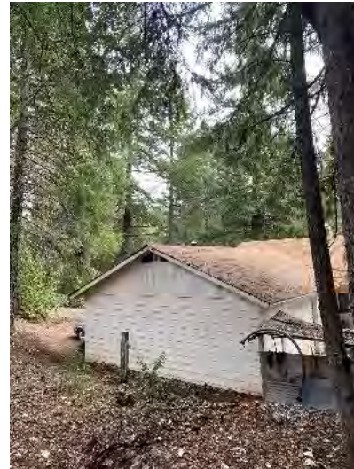
Photograph 3. Defensible space treatments are proposed in areas where tree limbs are located in close proximity to or are overlying existing structures.
