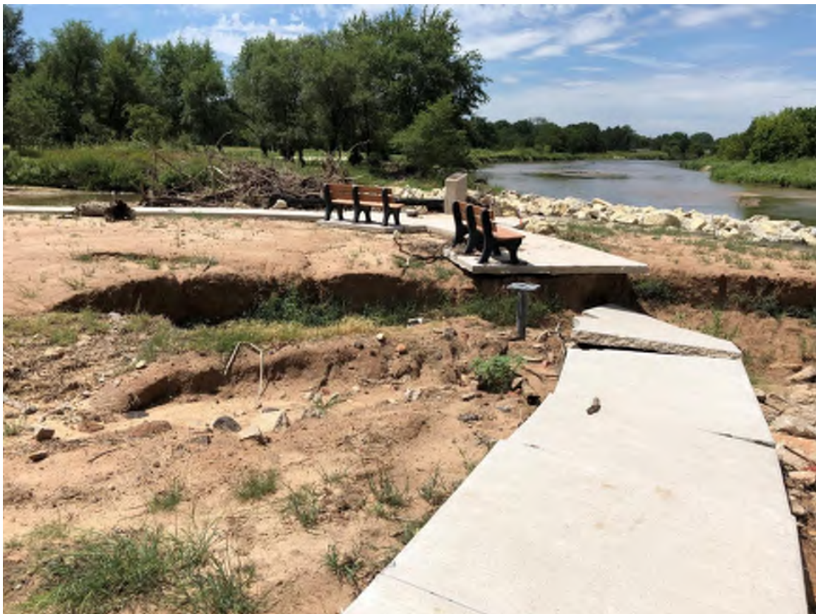
Figure 6: 2019 South Fork Ninescah River South Bank Damage Conditions
