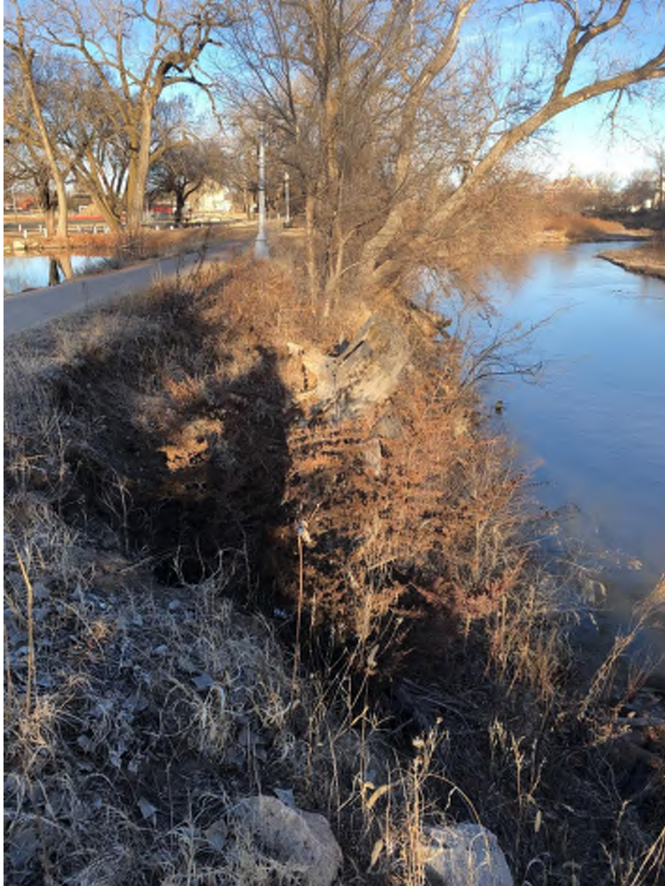
Figure 4: Ground Level Photo of the 2021 Slope Conditions
