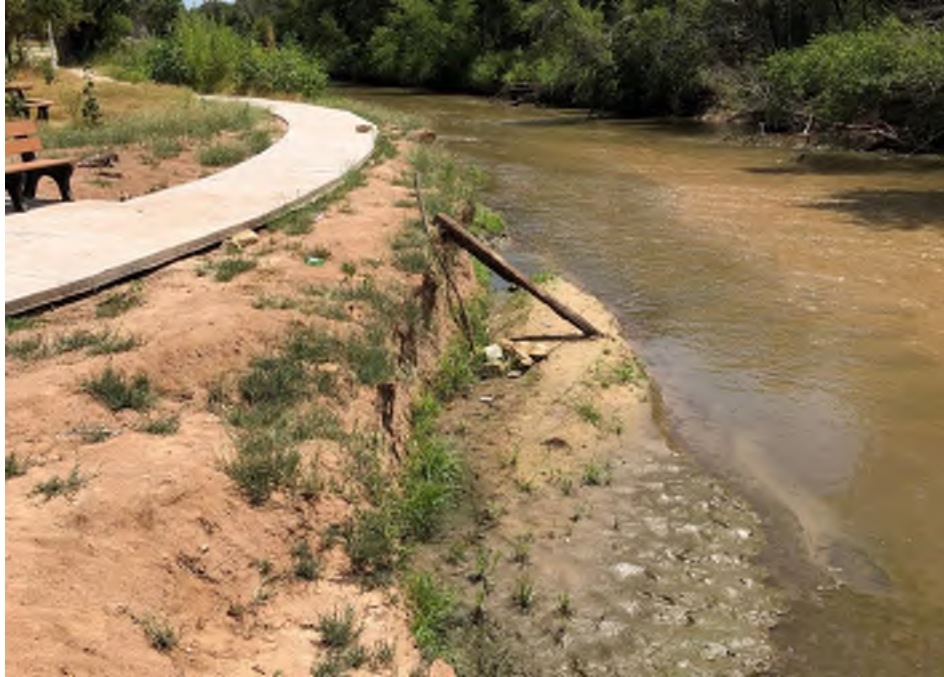
Figure 7: 2019 Mill Race North Bank Damage Conditions
