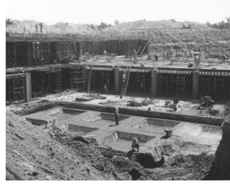
Construction of Federal Regional Center for Region VI in Denton, TX on August 31, 1962.
